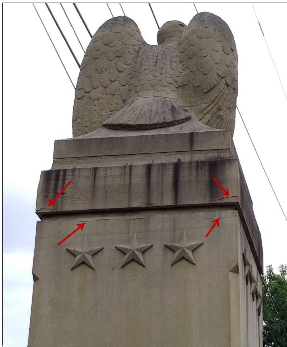
Photo 42: Detail of the south elevation of the northwest pylon showing the relatively minor stone deterioration at the sculpture. The degree of biological growth at the top profile block at this elevation is typical. Note also the delamination at the bottom of the top profile block and the top of the upper column block (arrows).
