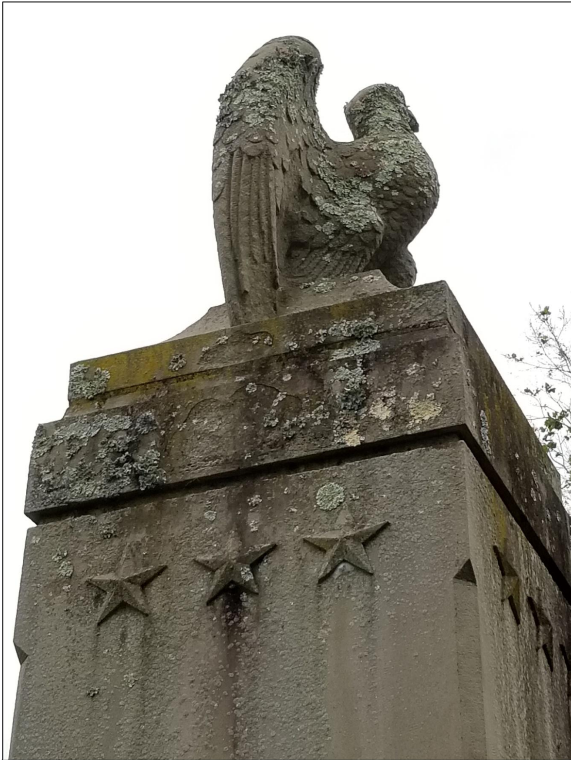
Photo 44: Detail of the east elevation of the northeast pylon showing the heavy accumulation of biological growth, particularly lichen.
