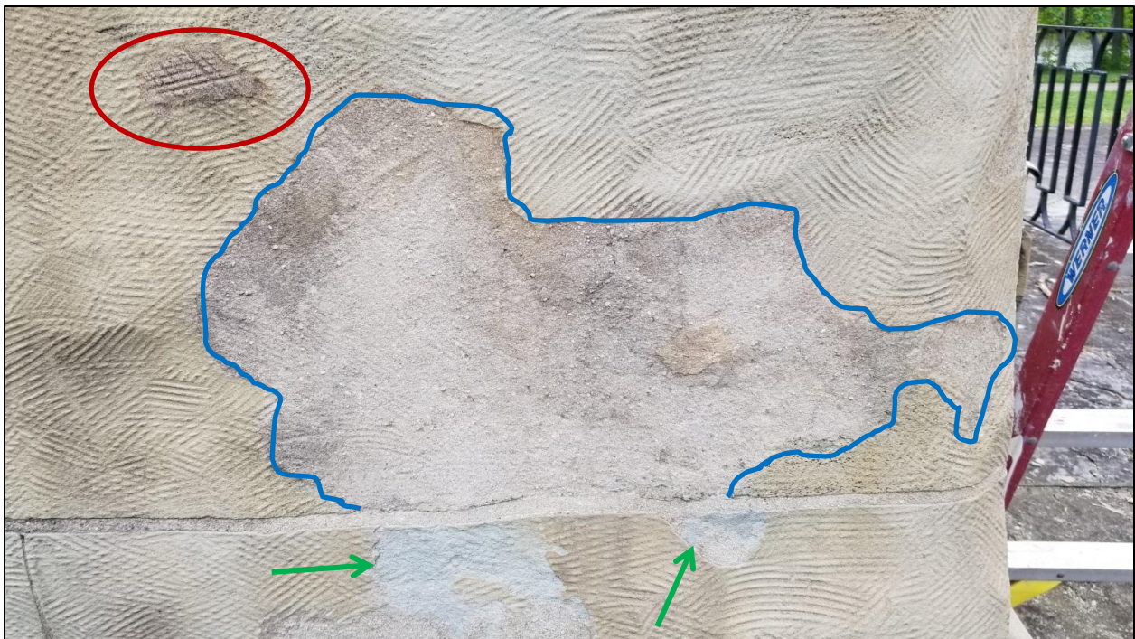
Photo 10: Detail of the lower right of the east elevation at the base showing two of the kinds of patching. The ceramic microspheres patching is circled in red (note the crude scratches in imitation of the chisel marks on the stone); the other patch type is roughly outlined in blue. Note the area below the joint and the large patch where the weathered yellow surface of the stone has been lost, revealing the blue color of the unweathered stone beneath (green arrows).
